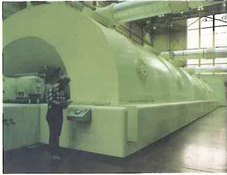
FIGURE 16-33 An example of a large steam turbine unit used in a nuclear power plant. Courtesy of New York Power Authority
